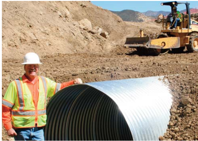
Road Maintenance Supervisor Steve Smotherman and his co-worker perform work to replace storm drain and road surface.
